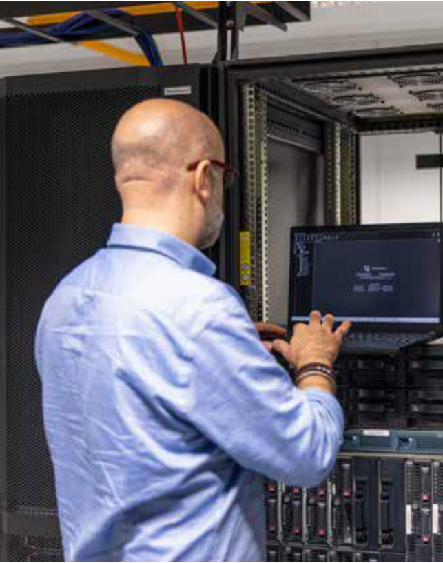
Smart Buildings e Data Centers
